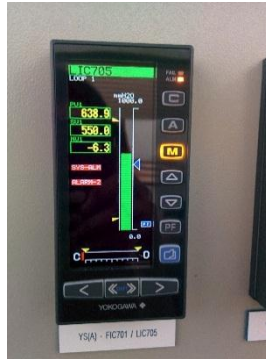
Gambar 2. 8 Display Boiler Drum
