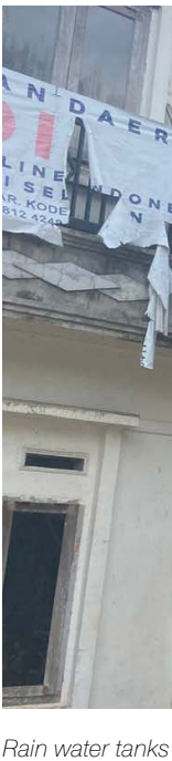
Rain water tanks
