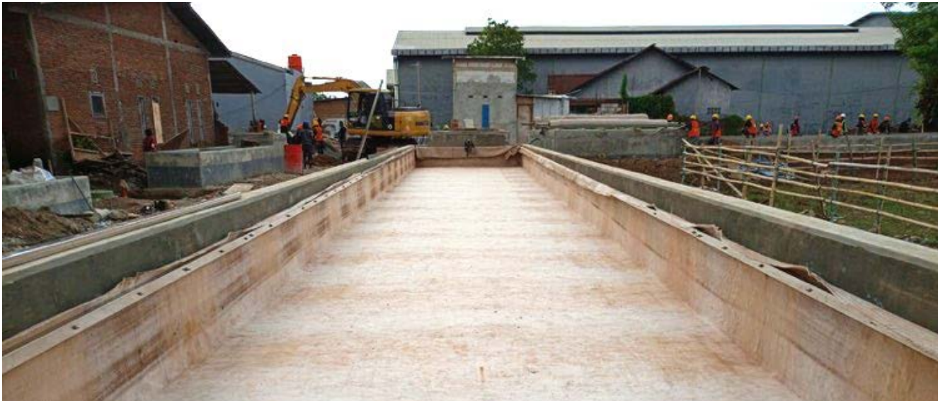
Septic tanks and wetlands
